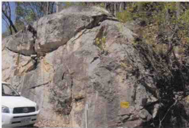
Culvert 188 - Drill marks on rock face
