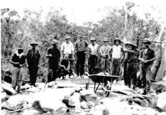
Figure 8 Road workers on Mt Spec Road (193?) Source: City Libraries Townsville, Local History Collection No. 0001/0001010.
