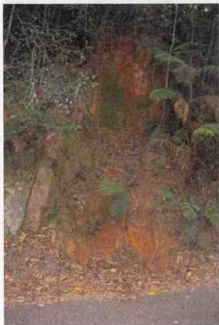
Culvert 46 - Large washout at inlet
