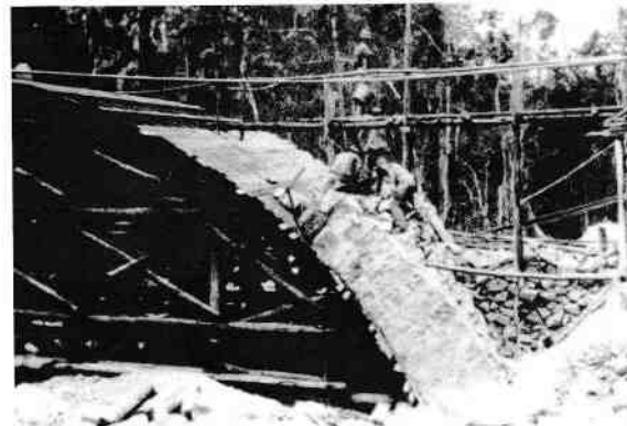
Figure 39 Abutment B (uphill end) of the bridge over Little Crystal Creek on 10 October 1932. Source: Qld State Archives Item ID 822274.
