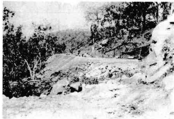
Figure 24 Construction of drainage on Mt Spec Road. Source: City Libraries Townsville, Local History Collection No. 0001/0001003.
