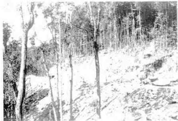
Figure 28 Construction of Mt Spec Road at the 11 mile peg Source: City Libraries Townsville, Local History Collection No. 0001/0001007.
