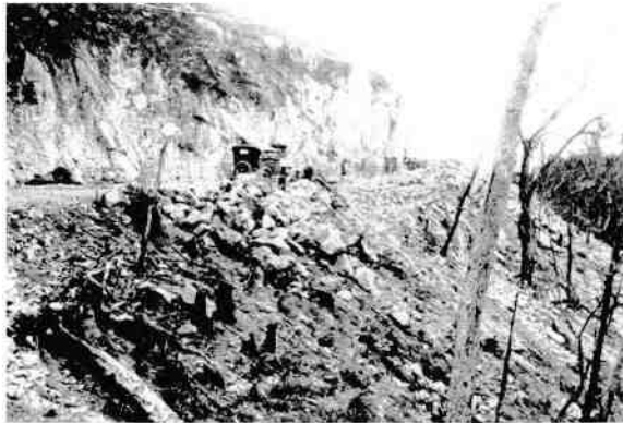
Figure 40 Stone cutting during construction of Mt Spec Road at 45,000 feet through chainage in c.1933. The car belonged to the McClellands. Source: City Libraries Townsville, Local History Collection No. 0000/0000999 and Venn, p.28.
