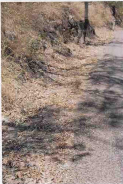
Culvert 198 - Intermittent stone kerbing and channeling
