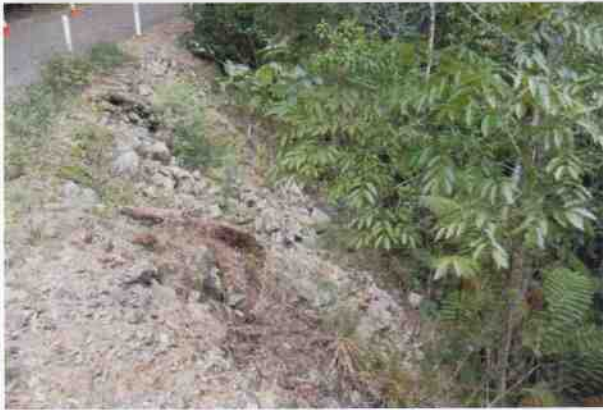
Culvert 58 - Rubble bank
