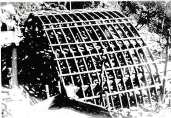
Figure 35 Formwork for Little Crystal Creek Bridge in 1932 Source: City Libraries Townsville, Local History Collection No. 0000/0000674.
