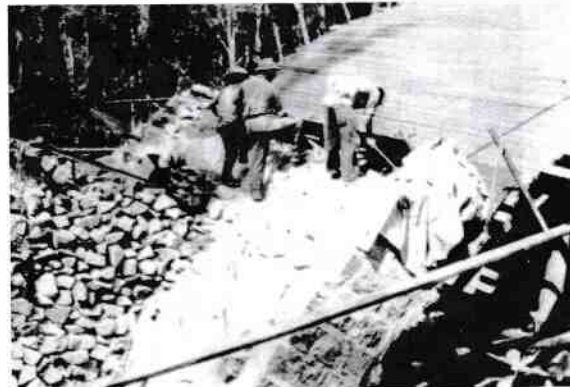
Figure 38 Abutment B (uphill end) of the bridge over Little Crystal Creek on 10 October 1932. Source: Qld State Archives Item ID 822274.
