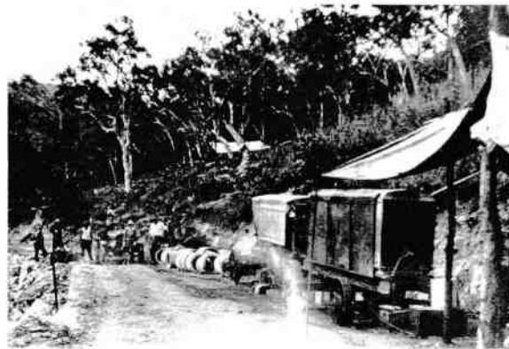
Figure 20 Tents, wagons and pipes on Mt Spec Road during construction (193?) Source: City Libraries Townsville, Local History Collection No. 0000/0000667.
