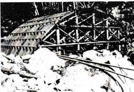
Figure 36 Formwork for Little Crystal Creek Bridge in 1932 Source: City Libraries Townsville, Local History Collection No. 0000/0000675
